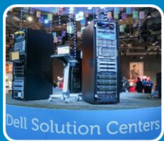
Data Center Management
